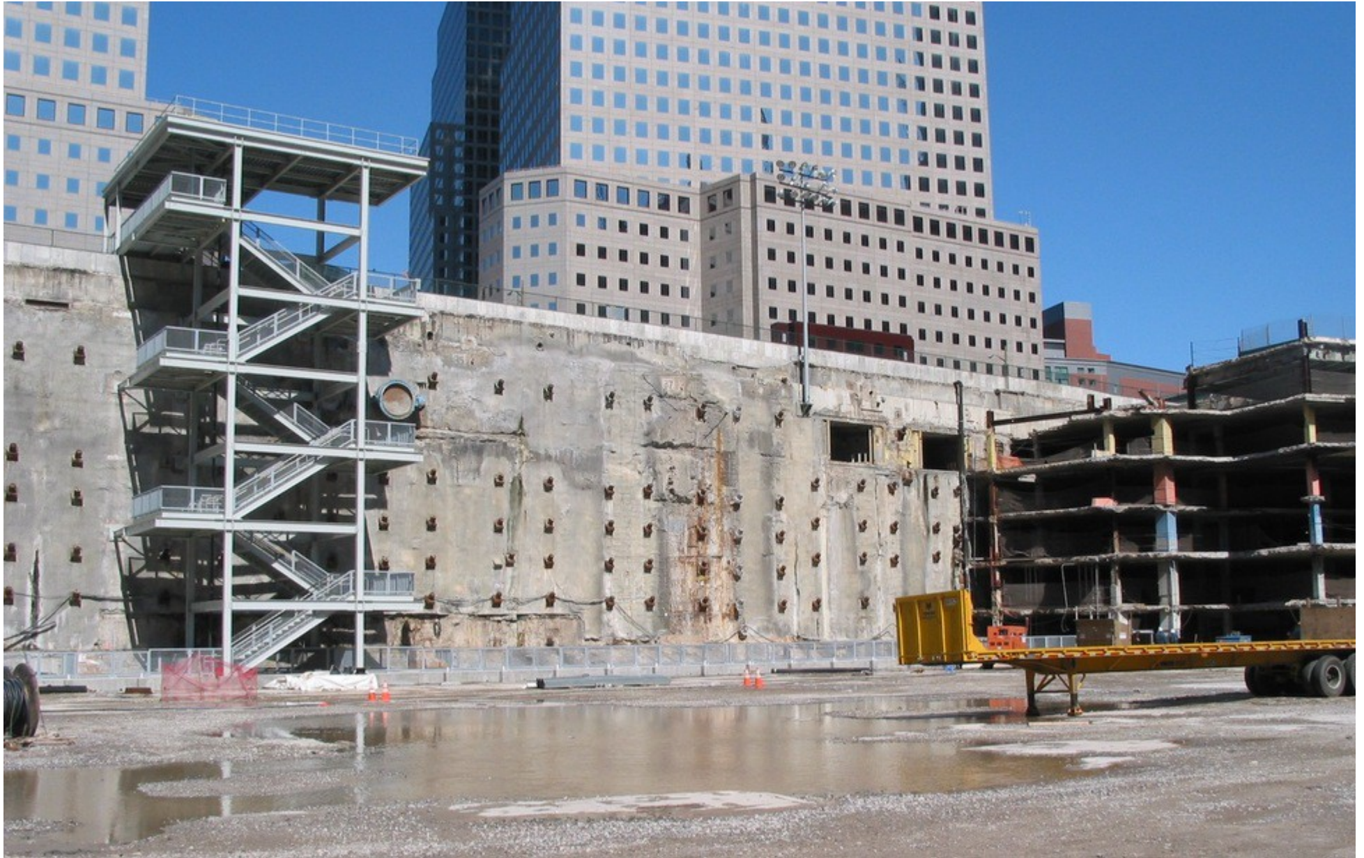
Figure 100. But, clearly the bathtub survived. This is a view from the footprint of WTC1. Notice the parking structure that was under WTC6 survived.
