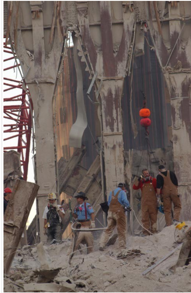
Figure 47. GZ workers walk in thick dust atop the rubble pile, hardly higher than the lobby level.
