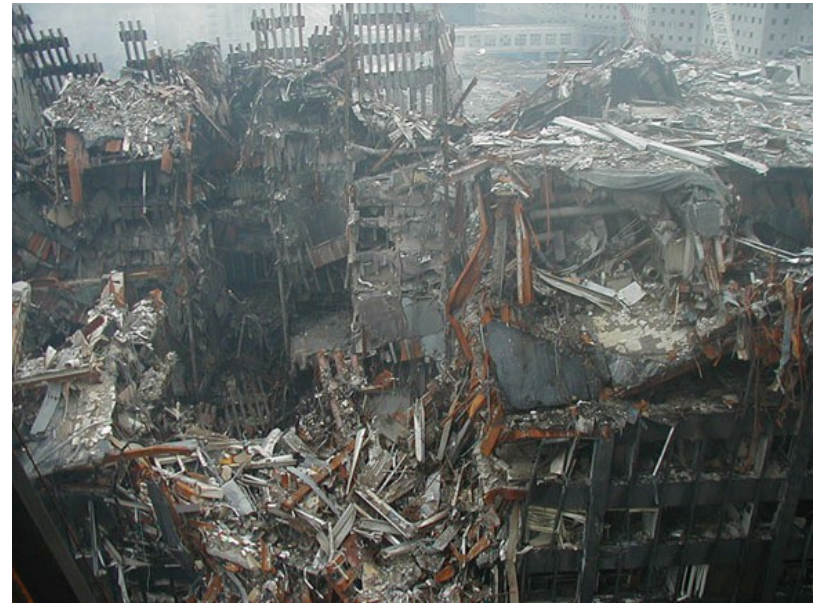
Figure 88(b). You can see the remains of WTC1 on the other side of WTC6. (WTC6 is in the foreground.) The amount of rust on beams adjacent to the hole in WTC6 is impressive.
