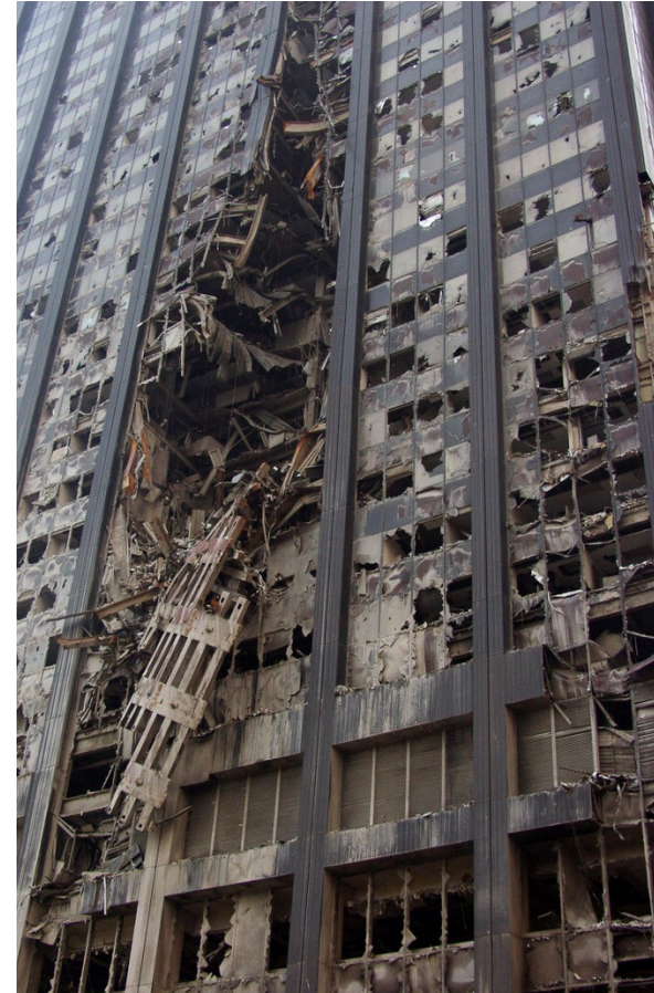
Figure 71. Bankers Trust Building on Liberty Street, across from WTC2. (FEMA picture)
