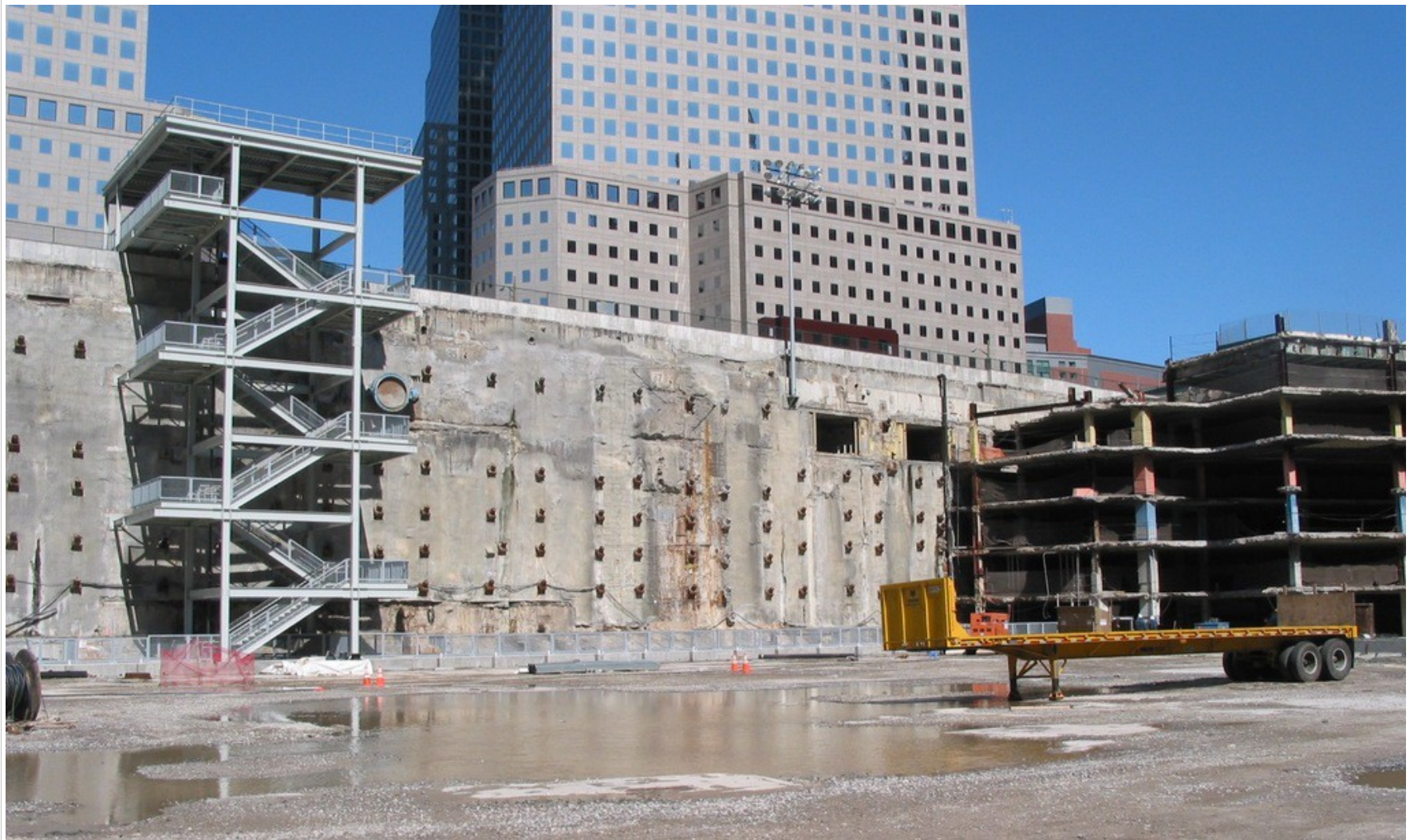
Figure 5. (old Figure 1.) There was no significant damage to the bathtub on 9/11. This picture looks west-northwest, from the center of the WTC 1 footprint.
